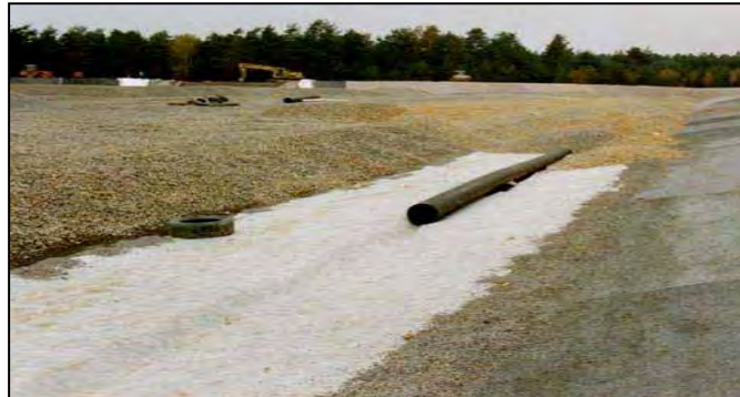
The drainage pipe for the leachate set on the geo-textile with an attached protection layer
